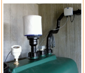
Biospüler storage tank with M422
